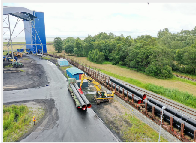
Shortly before completion: In mid-December, OGE connected the WAL pipeline to the German natural gas network via the North German Natural Gas Transversal (NETRA) pipeline. © OGE
