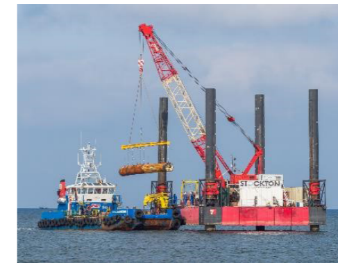
Figure 9: Direct Pipe® machine recovery after successful installation of a protection pipe for the export cable of the Beatrice offshore wind farm in Scotland
