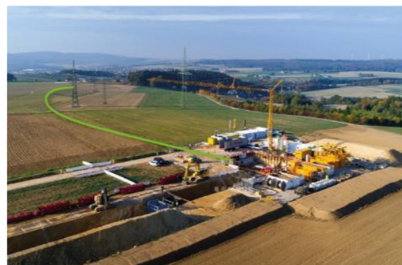
Figure 3: E-Power Pipe® in use in Bacharach for installing 6 parallel cable protection pipes, each with a length of up to 700 m
