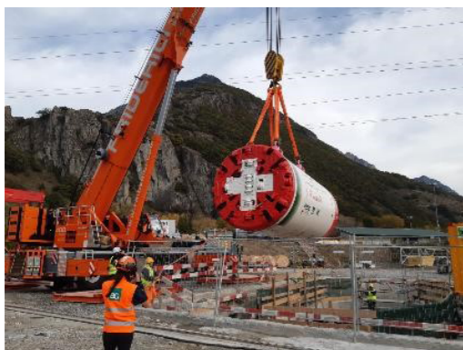
Figure 2: Construction company CSC Costruzioni, a subsidiary of Webuild, lowers the AVND 3000 into the launch shaft.
