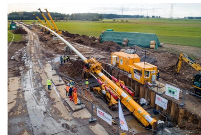
Figure 10: First Direct Pipe® system with jet pump technology on a DN 700 gas pipeline project GIPL in Poland.
