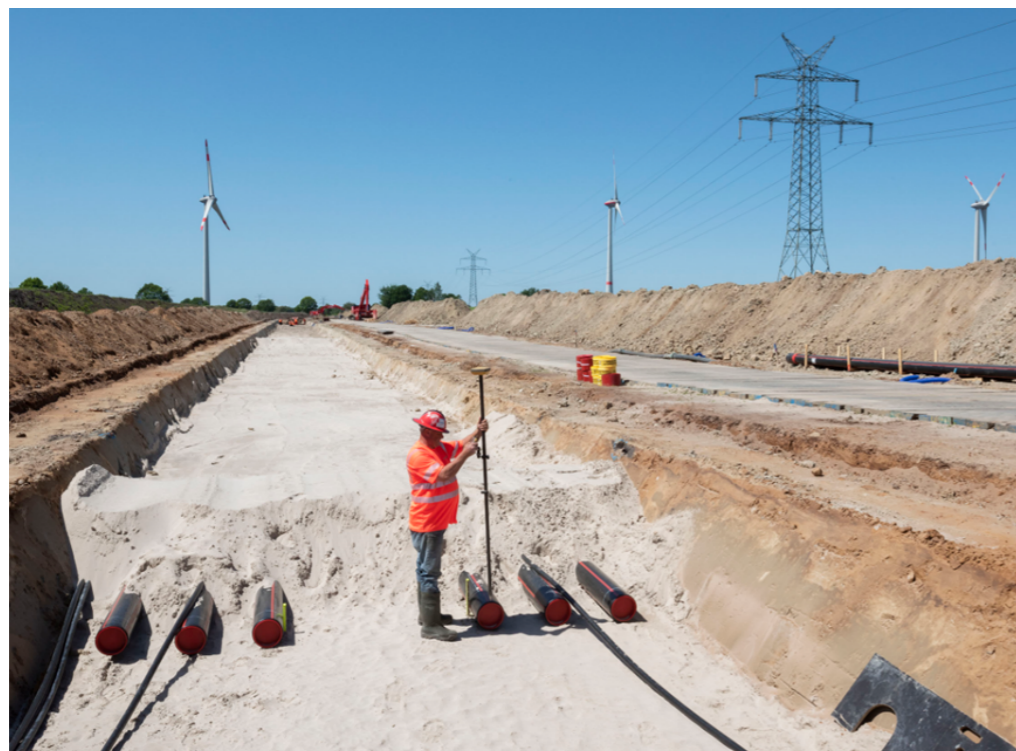
Figure 4: parallel laying of cable ducts 379 kV, replacement building in Emden-Ost Conneforde, source TenneT
