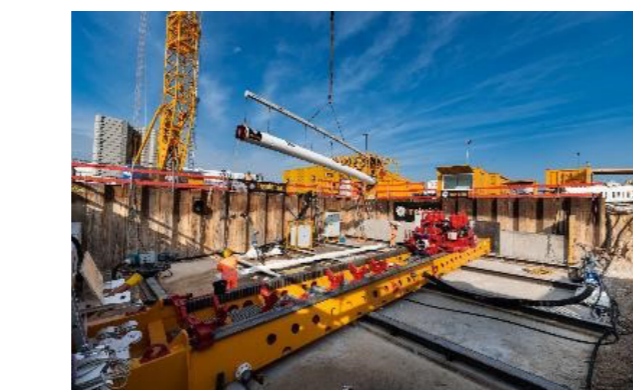
Figure 7: E-Power Pipe® installation in the launch shaft with AVNS350XB tunnel boring machine and rack-and-pinion jacking frame
