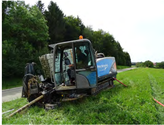
Fig. 10: Grundodrill 18ACS in permanent use, limestone only a few decimeters under the surface
