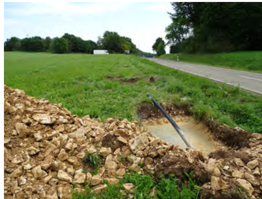
Fig. 11: Typical drill section parallel to road, protection pipe for fibre-bundles in the foreground
