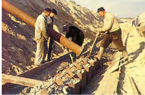
Fig. 2: Construction of a horizontal drain (with gravel pack) in a trench in the 1950's.
