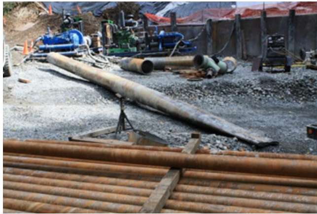
Installed casing pipe not strong enough
