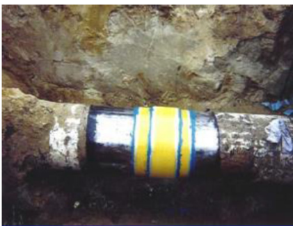
Composite repair (e.g. basis carbon fibre)
