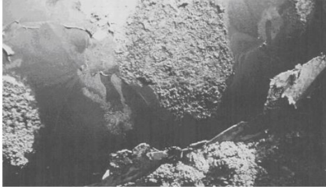
Figure 3.4 – Disbonded pipeline coating associated with external localized MIC. (Source: Peabody's Control of Pipeline Corrosion, 2 nd Edition, p. 274. Courtesy Dan Pope, Bioindustrial Technologies, Inc.)
